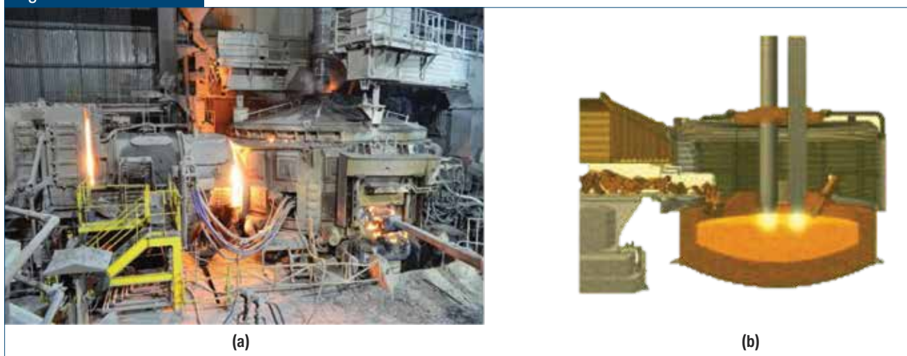
View of the EAF, lintel and Consteel conveyor at Nucor Steel-Hertford County (a) and section view of a Consteel EAF (b). 3
