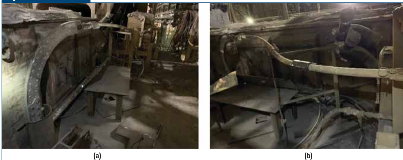
Picture of the CoreTemp installation on the EAF sump as viewed from the sanding hole (a) and picture of the CoreTemp installation on the EAF sump as viewed from the wire feeder (b).
